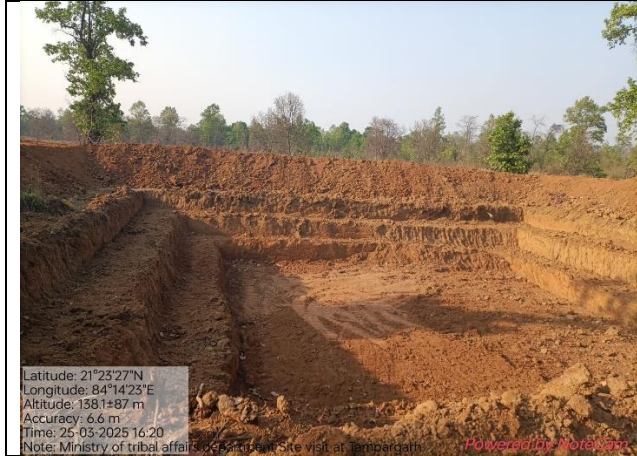
Percolation Tank at Dhalapal(PT),Sambalpur
